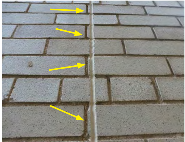
Photo 2 Poorly Aligned Remedial Expansion Joint
